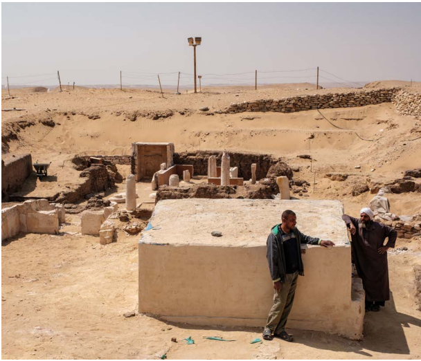
Fig. 37 New protection installed around the Ramesside chapel (context 270). Photo by Servaas Neijens, 2023/Leiden-Turin Expedition to Saqqara.
